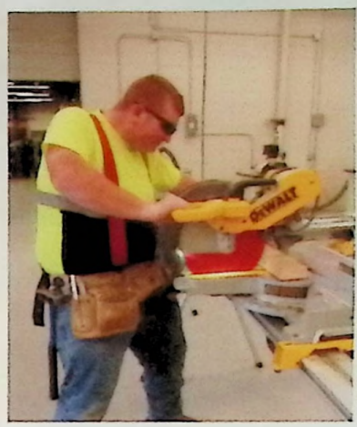
JAKE CARTER CAREFULLY MEASURES AND CUTS PIECES OF WOOD TO HELP BUILD THE NEW HOUSE FOR THE CARPENTRY PROGRAM.
