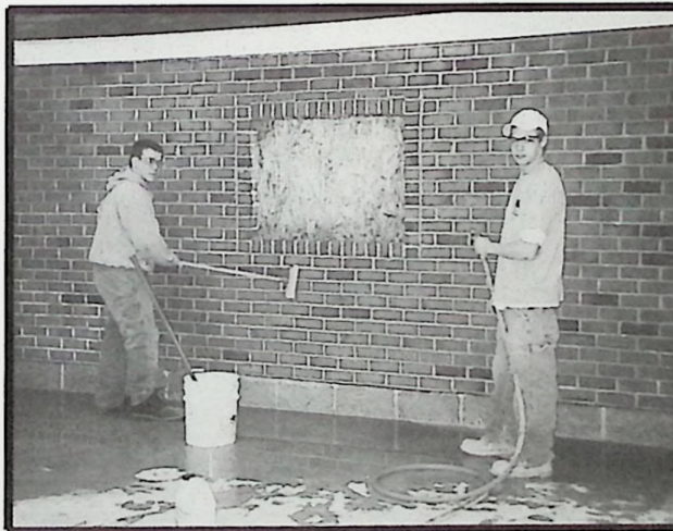
Nathan Thompson and Tyler Lilly clean a wall at Vocational School. The purpose of scrubbing the wall was to remove excess mortar.
